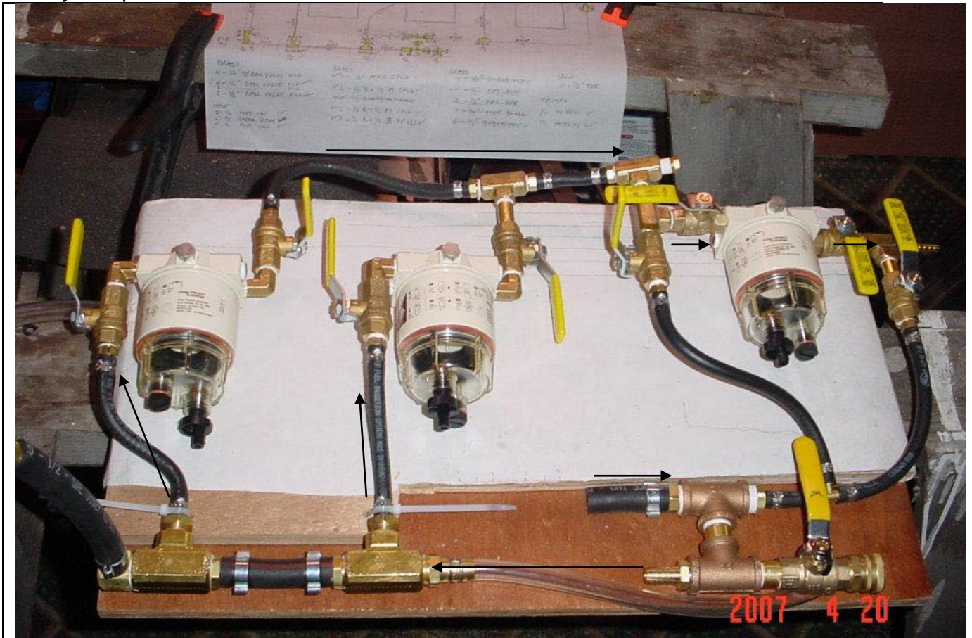
Duplex two-stage filter bank with bypasses. Filters were assembled on a mounting board in the shop. Arrows show fuel flow direction.
