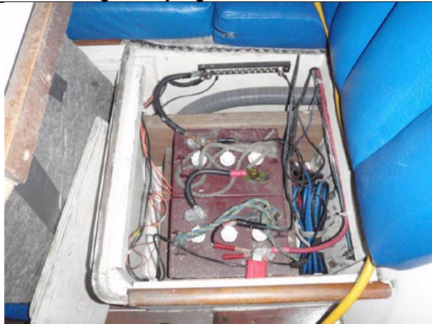
Dual 6 volt batteries in series.
